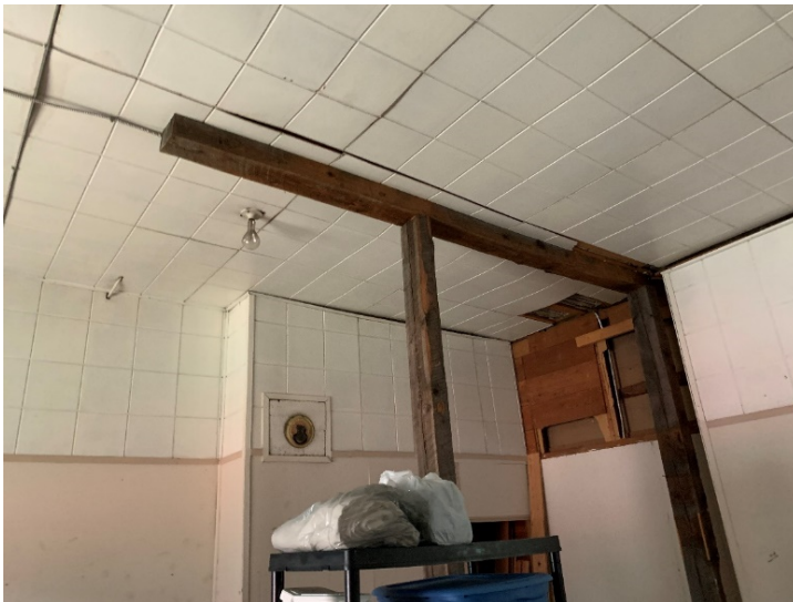
Photo 4: Post and beam propping with floor deflection evident in ceiling tiles
