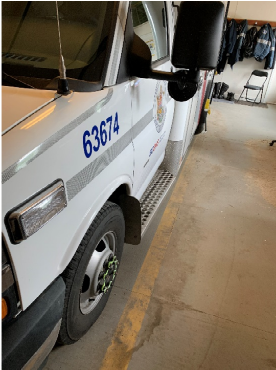
Photo 5: Water staining on sheathing around the ambulance
