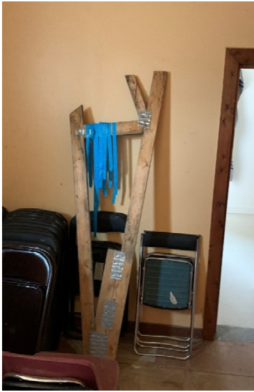
Photo 2: Cut roof truss on main floor
